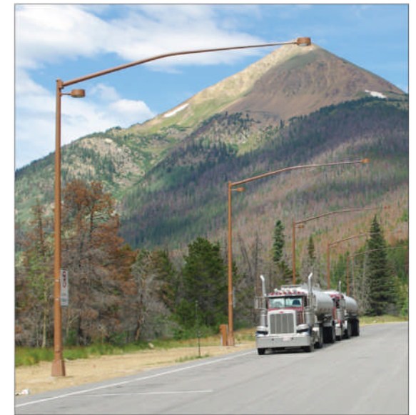
C | Concentrate lighting and utilize intelligent systems at major road service areas like the chain-up station at Watrous Gulch (EB & WB mm 219). The image above is an ideal example of forest service brown.
