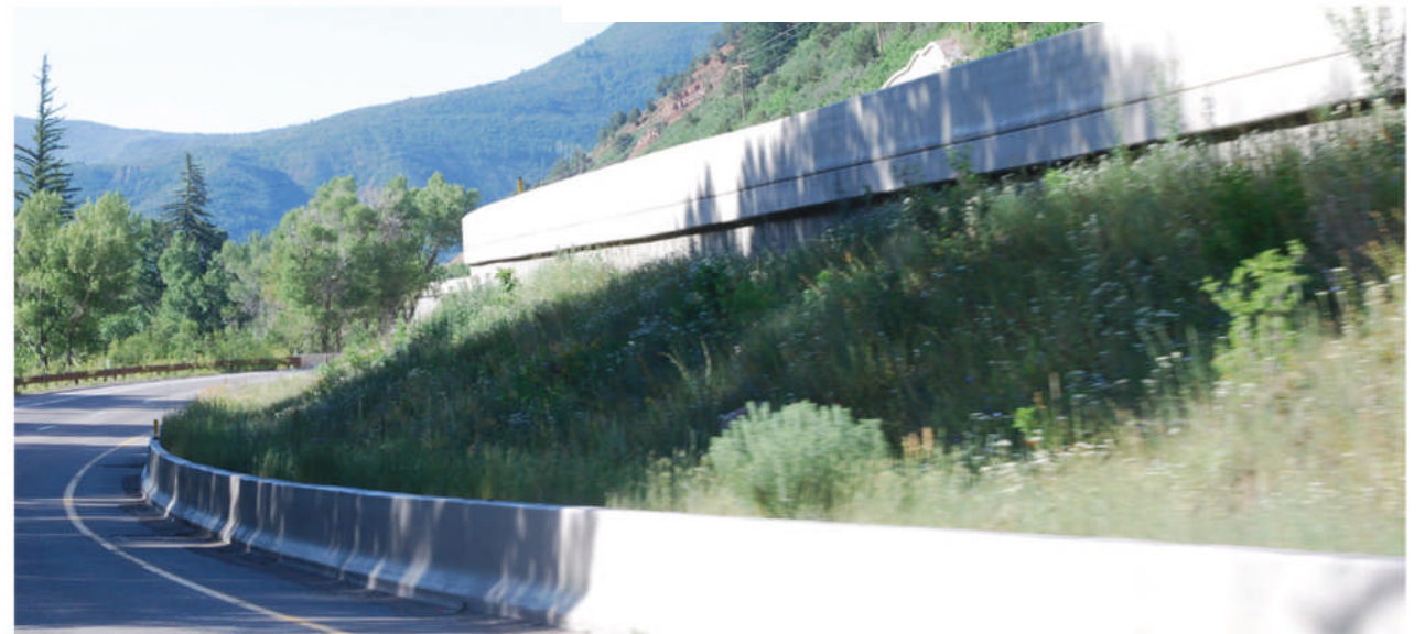
C | Continuous concrete barriers with a consistent color application should be utilized rather than segmented barriers.
